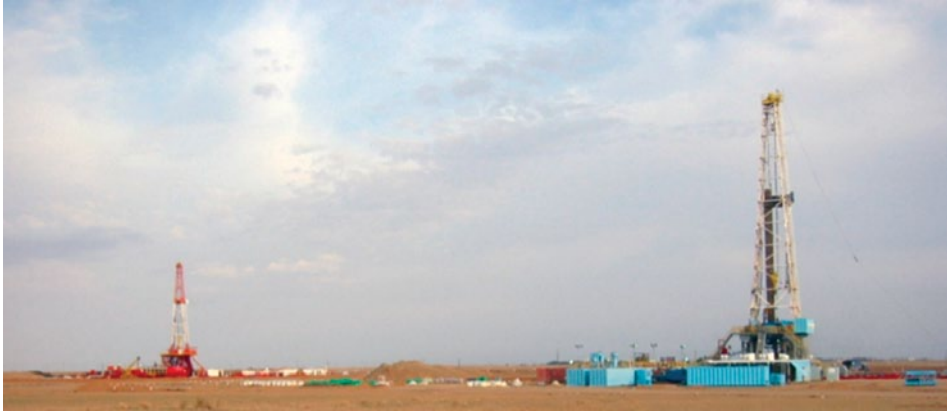
▼ Relief-well rig in foreground and problem-well rig in background (see page 14–15). Photo: add wellflow as
